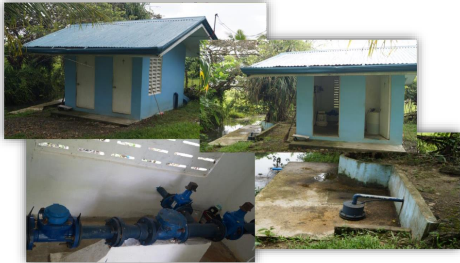
Figure 7. Omod Pumping Station Facilities and Spring Box
