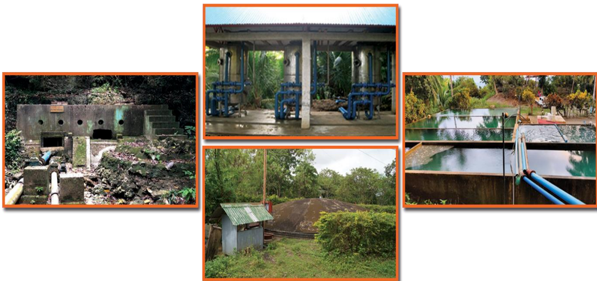
Figure 4. (Left) Spring Box; (Upper Center) Softener; (Lower Center) Muyoao Reservoir; (Right) Flocculation, Sedimentation, Filtration
