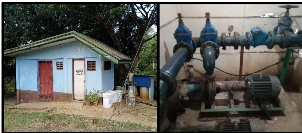
Figure 5. Cambulo Pumping Station and its facilities
