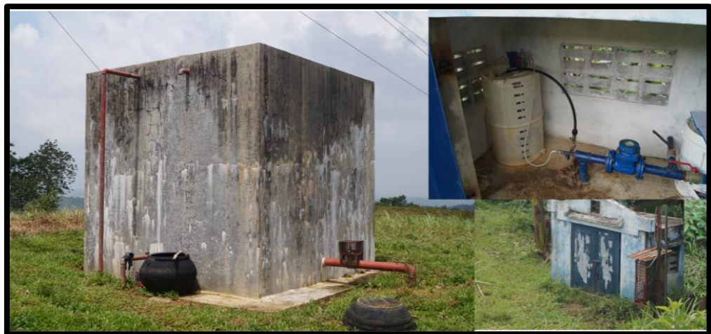
Figure 9. Dawis Spring Box and Pumping Station and Reservoir
